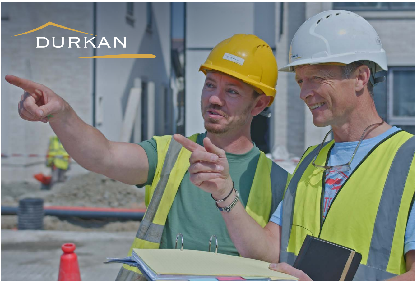
From the right: Neil Durkan on site at Fairfield with site manager Michael Hickey.
